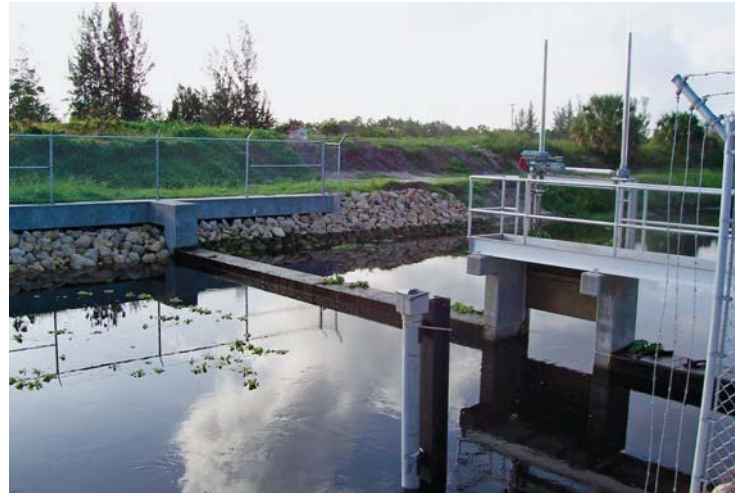
District water control structures are checked and serviced on a quarterly basis
